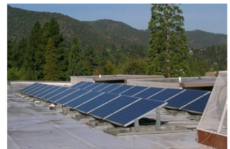
Solar PV array on the Hannon Library
